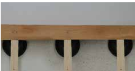
25. Position the first row of wood boards, screwing them to the underlying joists.
