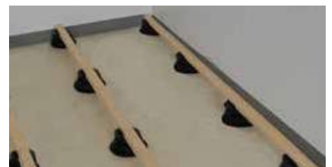
21. Check to make sure that the wood joists are firmly attached to each pedestal.
