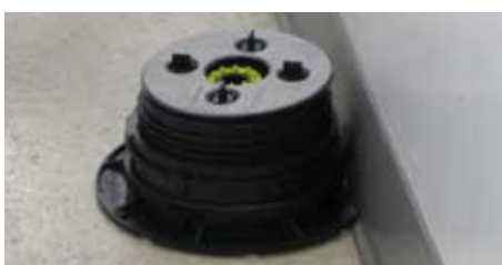
8. Assemble the pedestals and position them with the cut side towards the wall.
