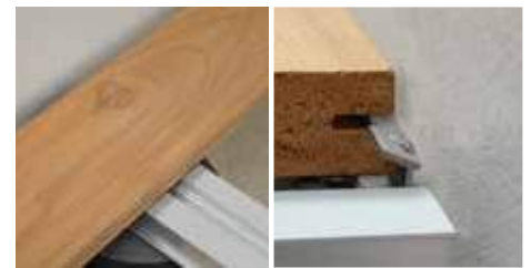
19. Install the first row of wood boards, inserting the groove into the SUPCLIP clip.
